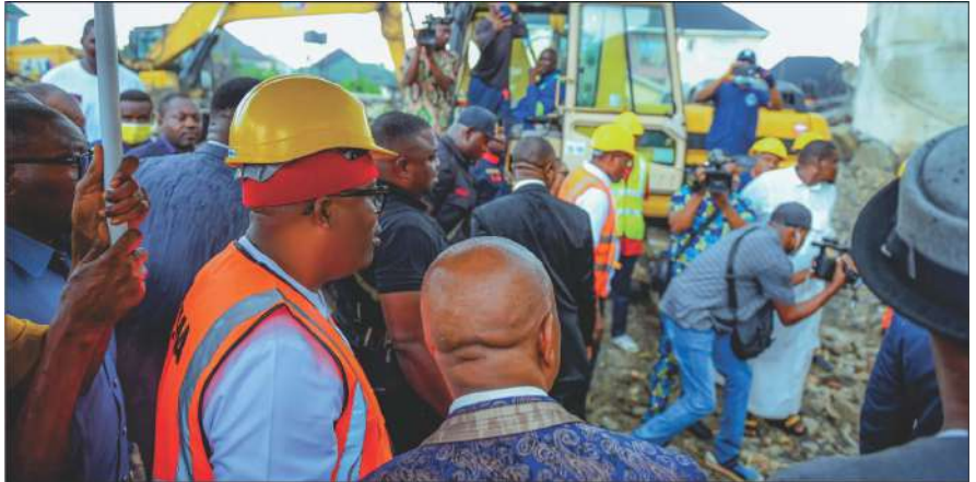
Gov. Sim Fubara of Rivers State and emergency rescue teams at work during evacuation operations following the building collapse in Port Harcourt, Rivers State.
