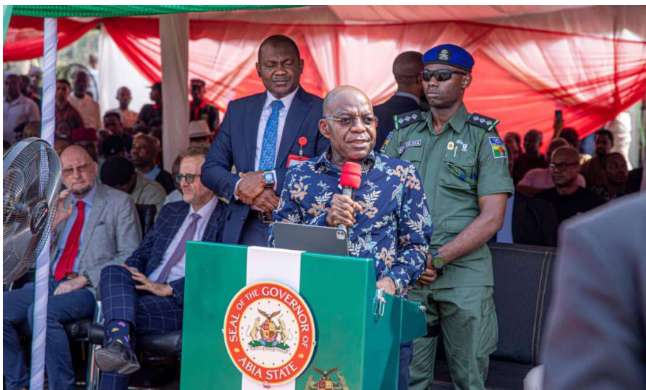
Abia State Governor, Dr. Alex Otti addressing Abian's during the flagged-off, reconstruction and dualization of the 5.5 kilometres Owerinta - Umuekea Road recently.
