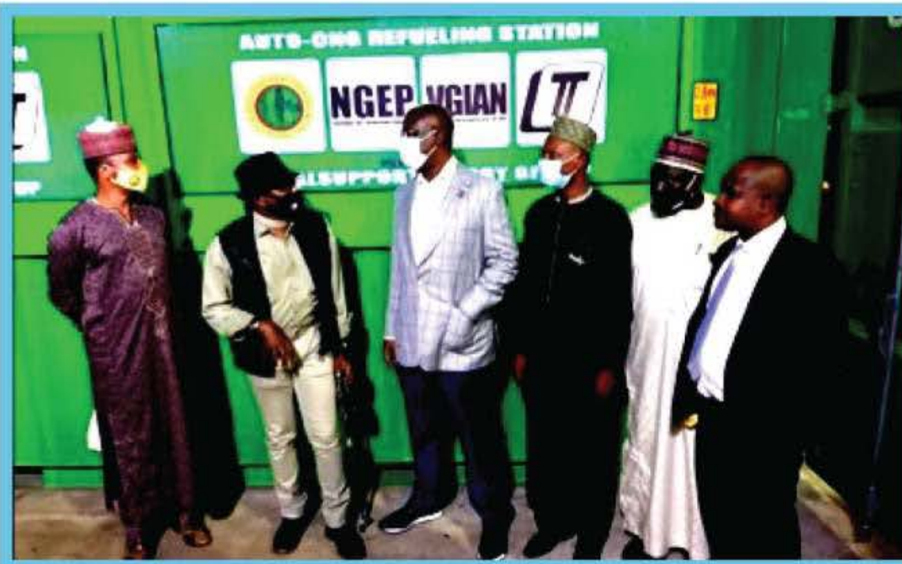
Hon Minister of State Tempre Silva inspecting our Containerized CNG Refueling Station
