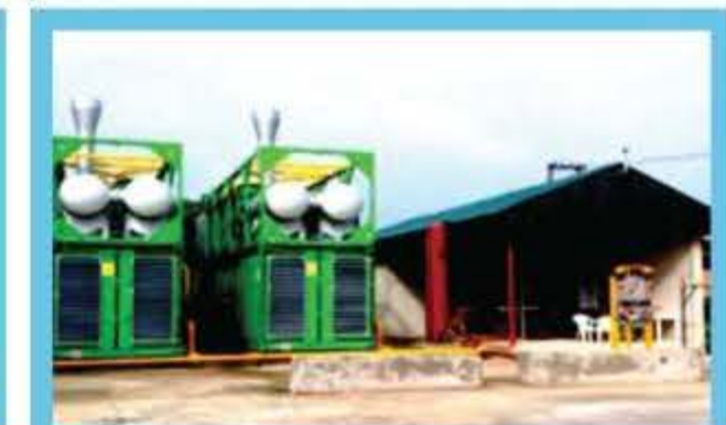
NGEP Power (CNG, LPG, LNG, ELECTRIC CHARGING) ISLANDS
