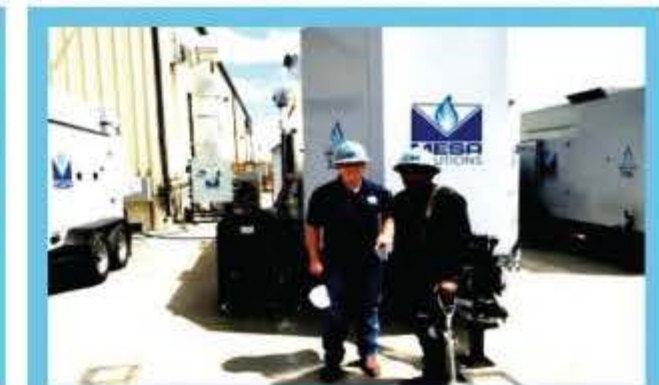
Customized MESA 350KW Mobile Gasgens
