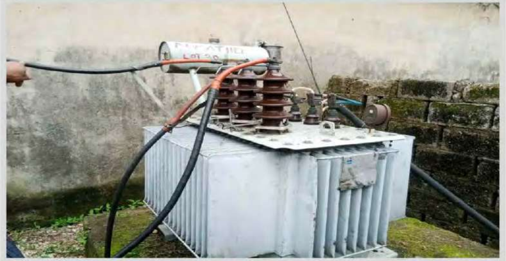
The repaired of the NEPA transformer that has been moribund for years by Rector Mr. Alloysius Ekeleme Okezie Administration
