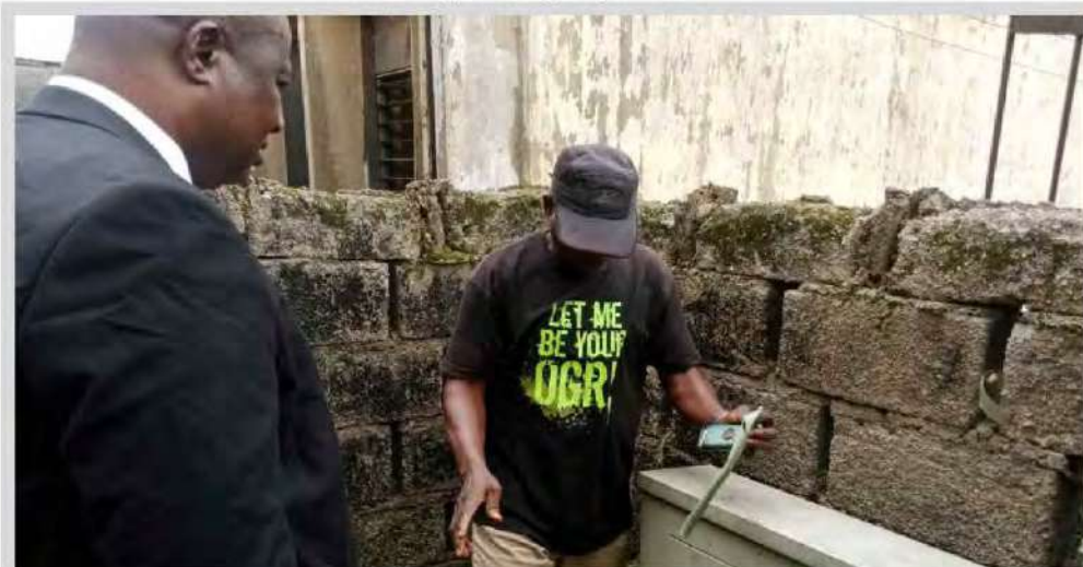
Evaluation of the repair of the NEPA transformer that has been moribund for years by Rector Mr. Alloysius Ekeleme Okezie Administration
