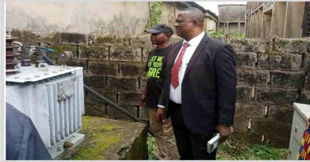
Evaluation of the repair of the NEPA transformer that has been moribund for years by Rector Mr. Alloysius Ekeleme Okezie Administration
